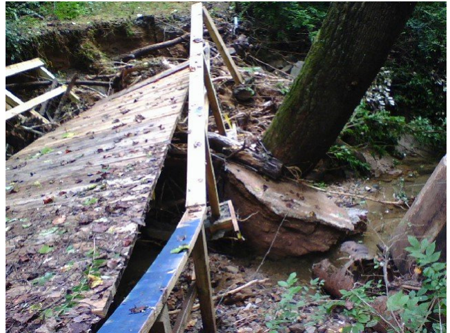
Bridge and culvert destroyed by storm to be replaced
